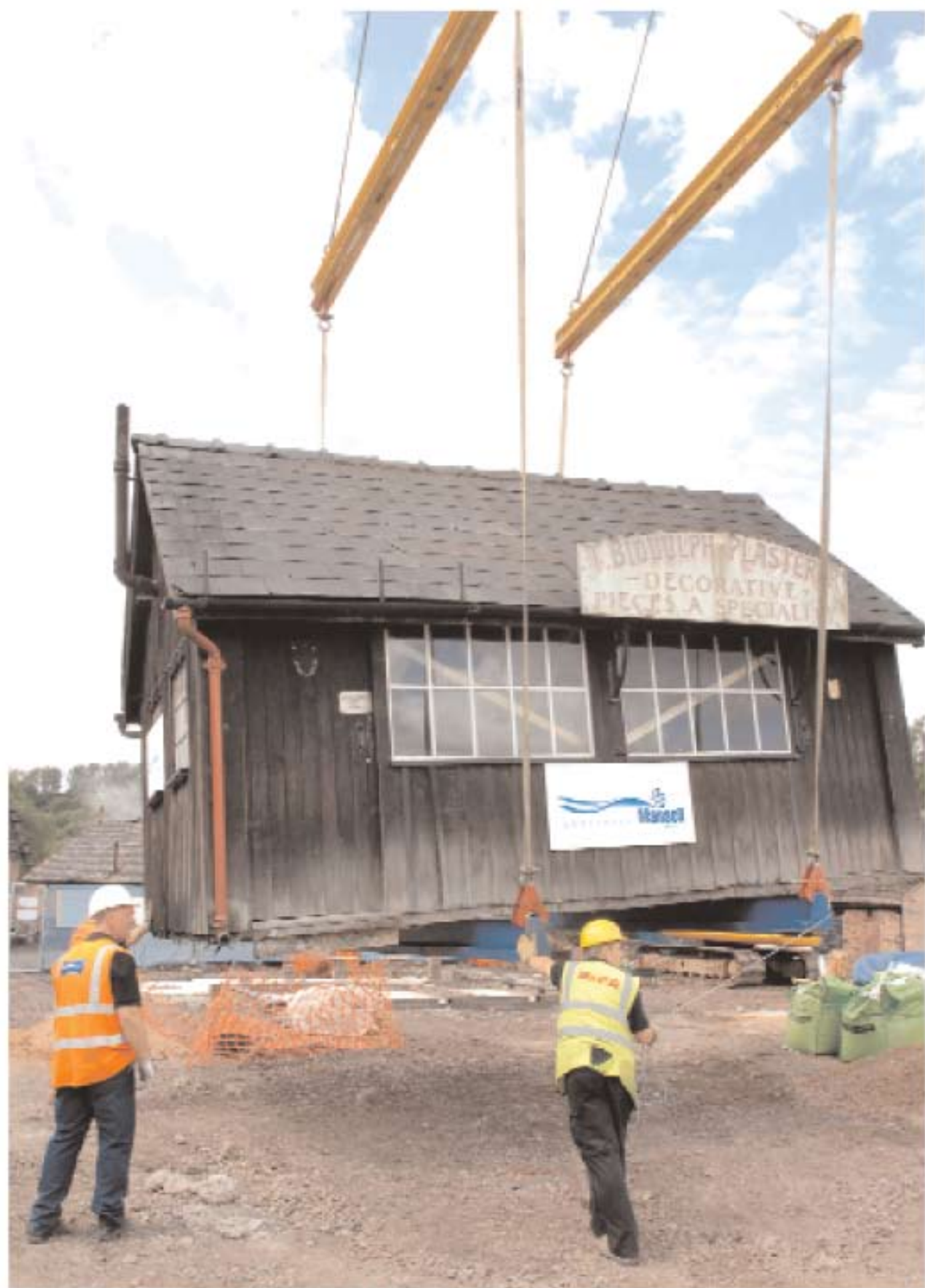
Building at Bliss Hill VICTORIAN TOWN makes headway with the moving of the Decorative Plasterer's Shop.
